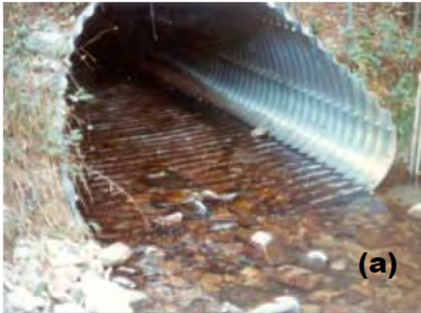
(a) Installed at-grade in 1979 for Fish Passage
