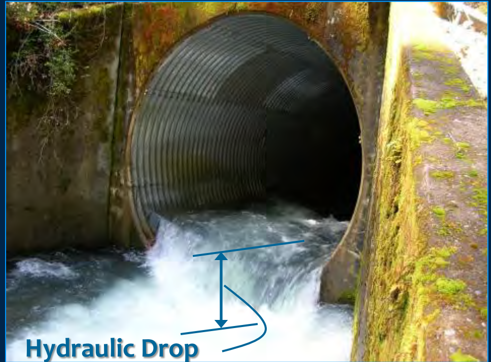
High Fish Passage Flow (excessive hydraulic drop)
