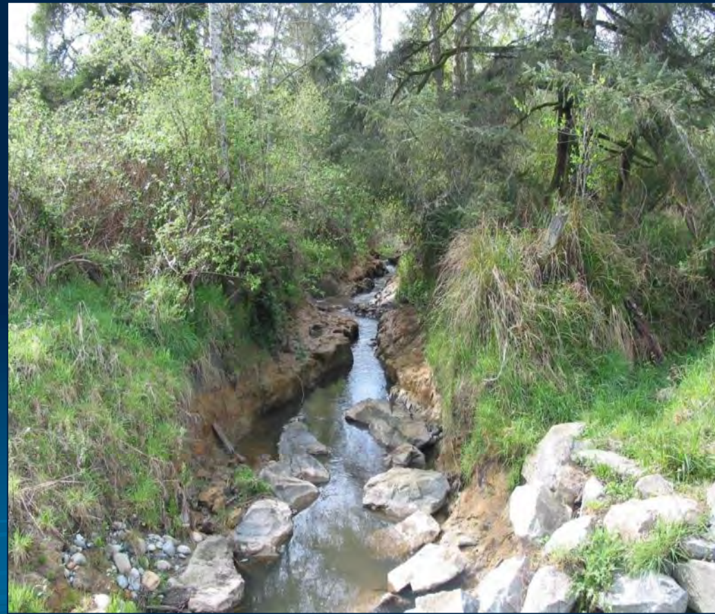
Upstream Incision after Crossing Replacement
