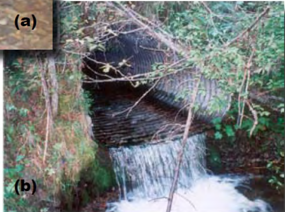
(b) By 1988 High Velocities from Culvert Caused Downstream Scour Pool and Outlet Drop
