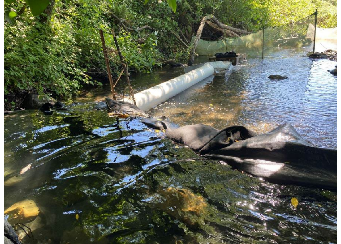
Dewatering pipe inlet
