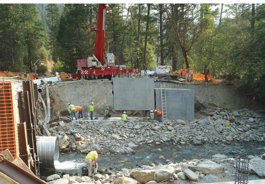
A cement slurry provided an excellent leveling pad for quick and accurate placement of 85-kip abutment segments.
